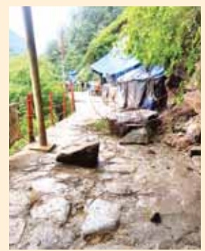
Debris lies on a road following a landslide on the Kedarnath trekking route, in Rudraprayag district, on Sunday. At least 3 pilgrims were killed and several others suffered injuries, according to officials. PTI
