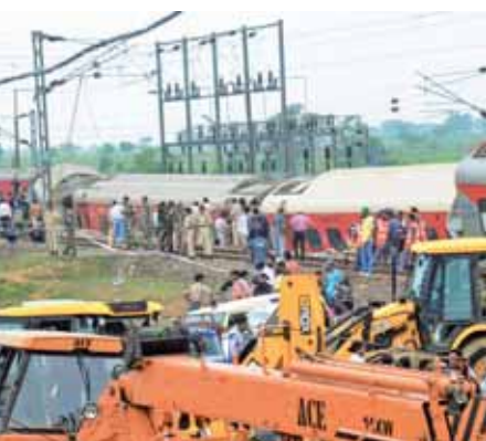
Rescue work underway after the Howrah-Mumbai Mail derailed near Badabambo, in Seraikela-Kharsawan district of Jharkhand, early Tuesday. At least two people were killed in the accident, according to officials PTI
