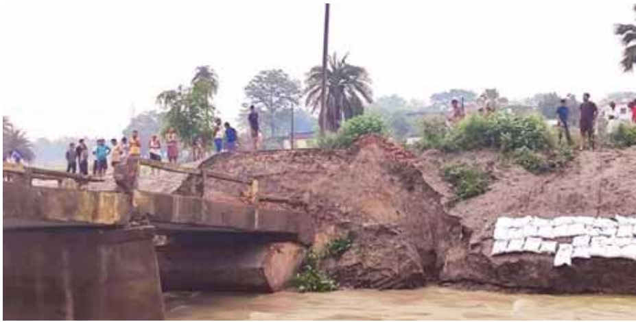
A view of the collapsed bridge amid heavy rain in Bihar's Siwan district on Wednesday
