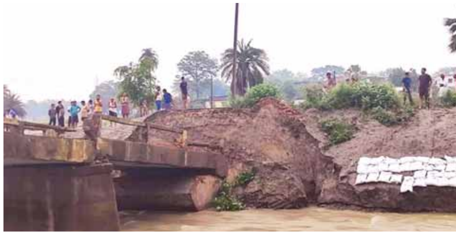
A view of the collapsed bridge amid heavy rain in Bihar's Siwan district on Wednesday
