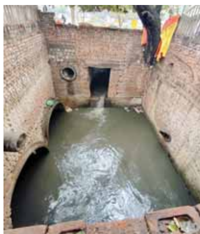
A dug up drain and an open drain near the Saket metro station
