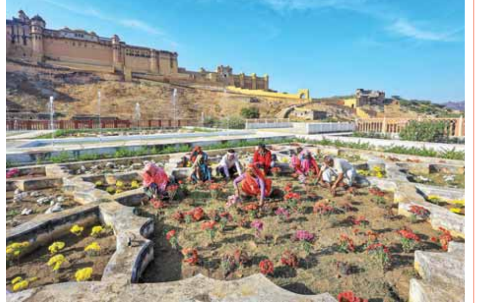
Beautification work in progress ahead of the Rising Rajasthan Global Investment Summit, at Kesar Kyari Garden of historical Amber Fort, in Jaipur PTI
