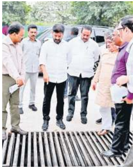
Chief Minister A Revanth Reddy inspecting the ongoing construction of a rainwater sump near Lake View Guest House on Hyderabad on Monday
