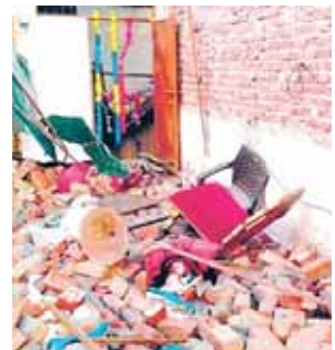
Eyewitnesses feared that a cylinder might have exploded, triggering the building's collapse and subsequent fire. However, after a thorough inspection, authorities confirmed that there had been no cylinder blast. Instead, the collapse was caused by the roof's failure, and the rupture of the PNG gas pipeline led to the fire. The six injured family members were rushed to Raja Harishchandra Hospital for medical treatment. According to doctors, they sustained a combination of injuries from the falling debris and burns caused by the proximity of the fire. Raju, the father, suffered 52 per cent burn injuries, while his wife Rajeshwari and son Rahul sustained 45 per cent burn injuries each. The three daughters, Mohini, Varsha, and Mahi, suffered burns to 50 per cent, 6 per cent, and 8 per cent of their bodies, respectively. The police are continuing to investigate the cause of the collapse and the fire.
