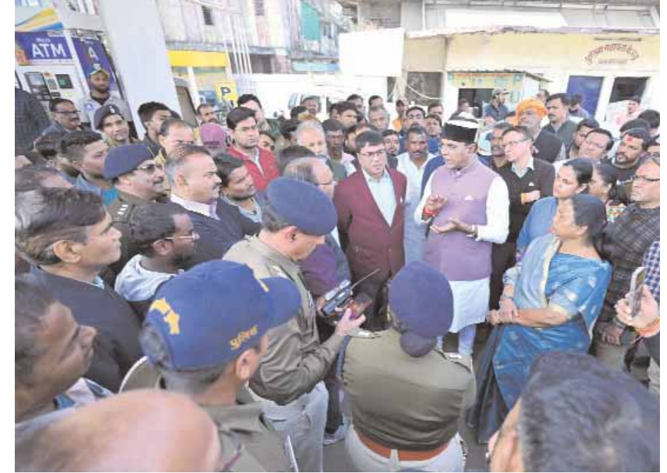
Minister for Sports and Youth Welfare Vishwas Kailash Sarang inspects under-construction road and drainage at Alpna trisection in Bhopal on Saturday.
