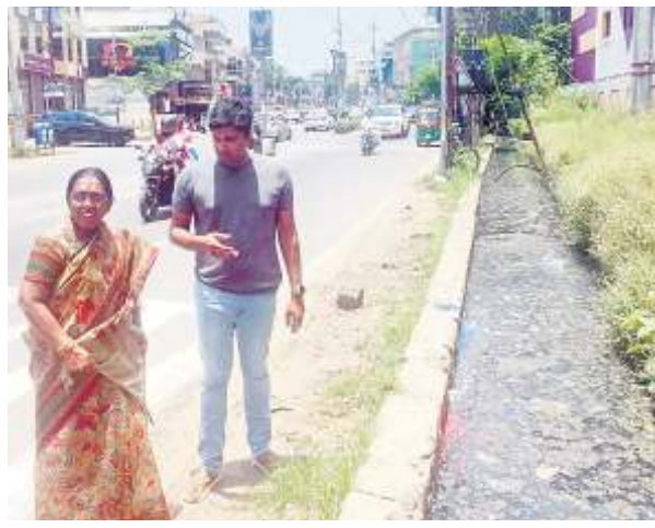
VMC Commissioner HM Dhyanaachandra, along with Executive Engineer Samrajyam, inspecting the side drain on the Pinnamaneni Polyclinic Road at Mogalrajapuram in Vijayawada on Sunday
