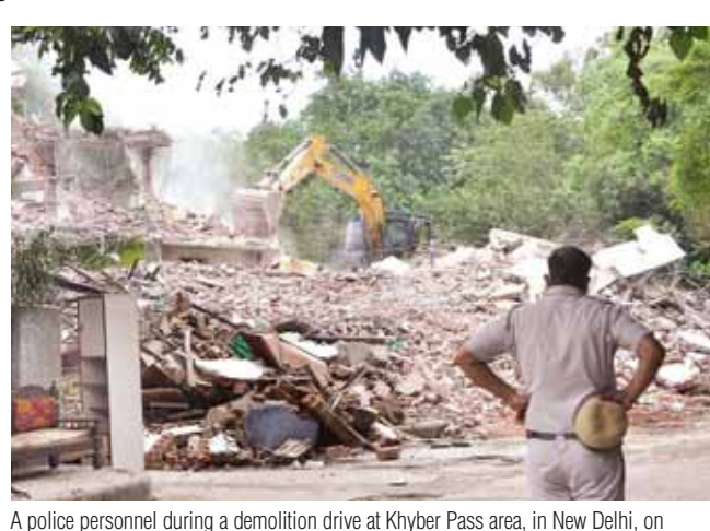
A police personnel during a demolition drive at Khyber Pass area, in New Delhi, on Sunday Ranjan Dimiri/Pioneer
