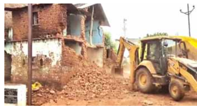
Rescue work underway after a wall collapsed at Shahpur village, in Sagar district, on Sunday PTI
