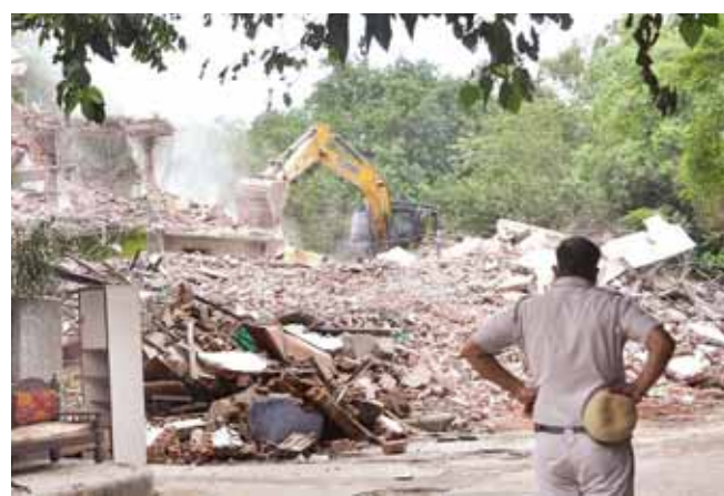
A police personnel during a demolition drive at Khyber Pass area, in New Delhi, on Sunday Ranjan Dimiri/Pioneer
