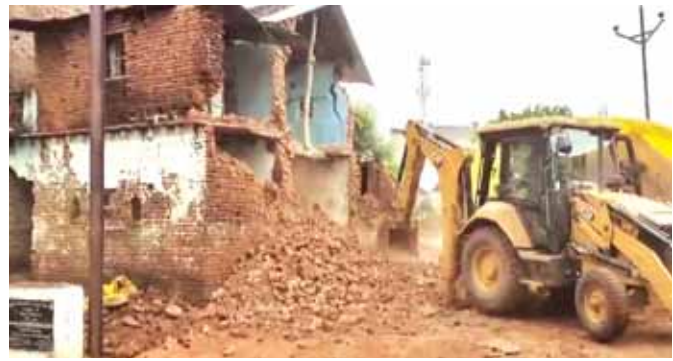
Rescue work underway after a wall collapsed at Shahpur village, in Sagar district, on Sunday
