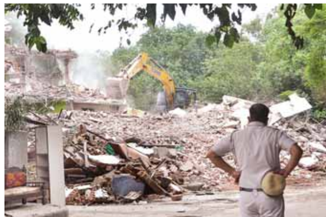
A police personnel during a demolition drive at Khyber Pass area, in New Delhi, on Sunday
