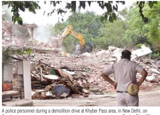
A police personnel during a demolition drive at Khyber Pass area, in New Delhi, on Sunday Ranjanj Dimiri/Pioneer
