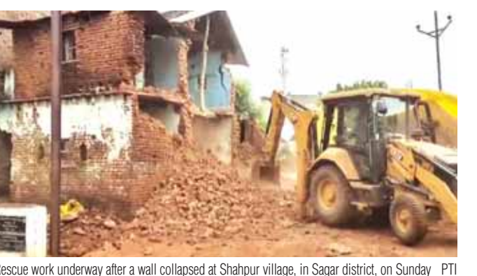
Rescue work underway after a wall collapsed at Shahpur village, in Sagar district, on Sunday PTI
