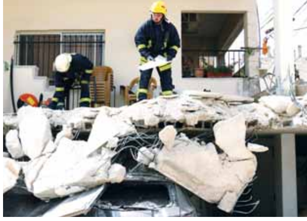
Palestinian civil defense workers clear the rubble from a damaged house following an Israeli military operation in the West Bank refugee camp of Nur Shams, Tulkarem, Friday. AP/PTI
