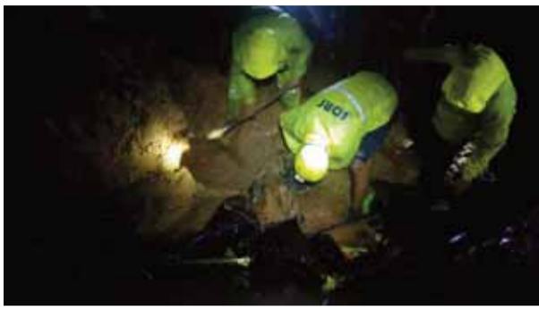
rescue team could not take a mechanical excavator to the site of the incident as heavy rainfall made the road inaccessible for heavy vehicles.
