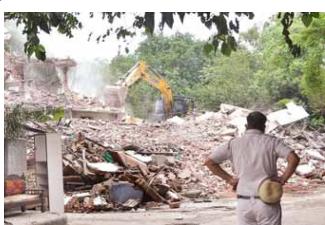
A police personnel during a demolition drive at Khyber Pass area, in New Delhi, on Sunday Ranjan Dimiri/Pioneer
