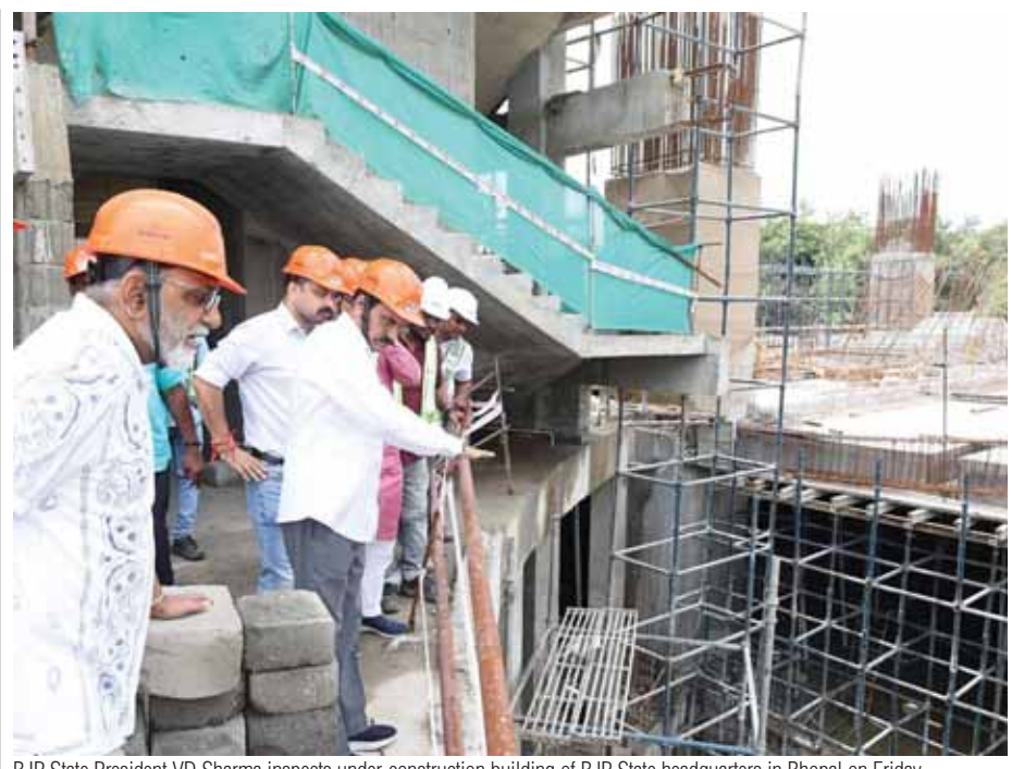
BJP State President VD Sharma inspects under-construction building of BJP State headquarters in Bhopal on Friday. Pioneer photo
