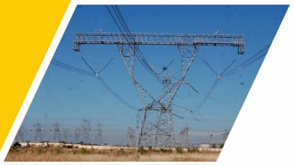
1200 kV Highest Voltage
